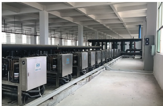
Large-scale green air-conditioning system
