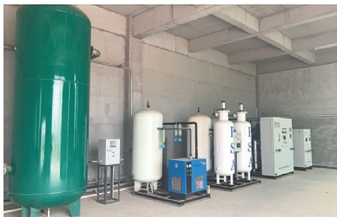
Purified Nitrogen system
